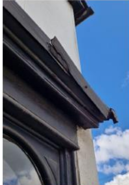
Figure 12. Damage to historic building in the conservation area as a result of passing large vehicles on the very narrow street.
